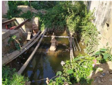
Leakages at the OHT
