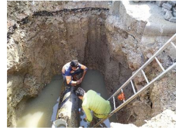
Water losses in pipelines
